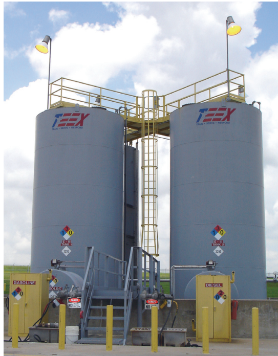
Figure 4.1: Cone Roof Storage Tank
